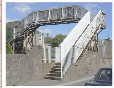
Before MSD Refurbishment
